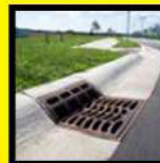
Storm Water Drains
